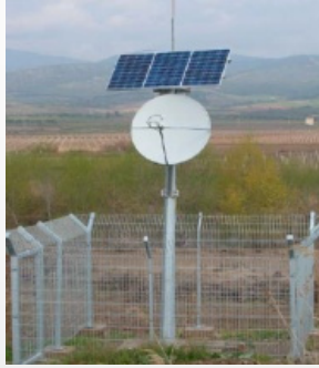
VSAT (satellite communication)
